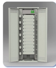
Optical Distribution Frame
